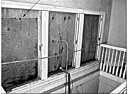
9 Missing historic windows (refer to window schedule) Repair damage to crown molding and plaster wall
