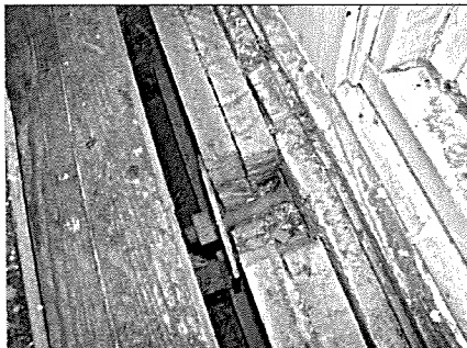
14 Beam damage from existing Fire Escape (Fire Escape anchor bolts)
